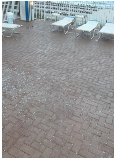
Thousands of little shards of glass on pool deck and between pavers.
